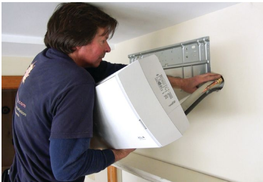
Chris Blaisdell of ReVision Energy mounts an indoor unit in a finished basement. Compared with the blower needed to move air through a ducted system, the small fan in this unit uses very little electricity.
