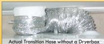
Actual Transition Hose without a Dryerbox
