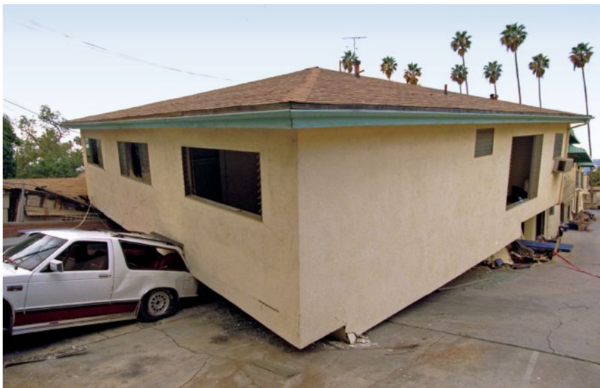
In an earthquake, shear walls help upper stories stay connected to the foundation, which moves rapidly back and forth. Without them, the movement gets too far out of sync, and the building "pancakes," as in this 1994 photo from Northridge, Calif.
