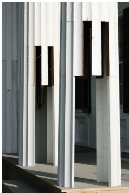
Figure 3. Starting with a long piece, five to seven custom-cut staves were installed on either side of a temporary 2x12 support, which was then removed so the final staves could be installed. Each segment joint was edge-glued with Titebond II and clamped with stainless steel screws driven at an angle every 15 to 20 inches.
