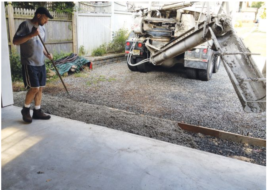
Figure 9. The apron slab was reinforced with wire mesh and sloped down toward the driveway 1 inch over its 4-foot width.
