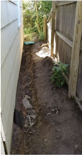
Figure 1. A teardown would have prompted the relocation of the new garage some 9 feet further into an already-small yard to accommodate the town's side-setback requirement of 12 feet.
