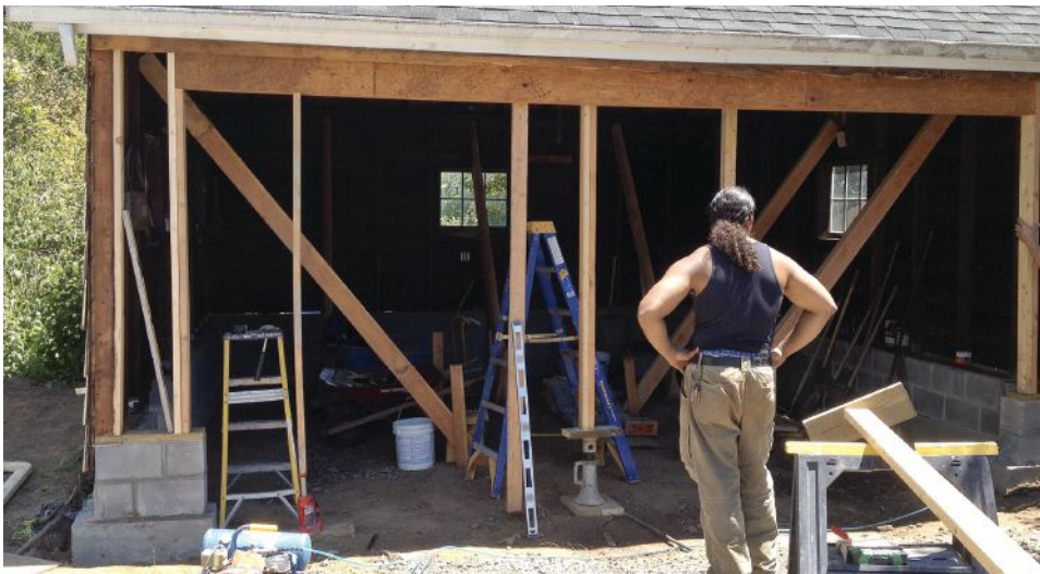
Figure 7. The wider overhead door required the installation of a double 11 7 / 8 -inch-deep Microllam header under the existing 4x4 top plate. A screw jack was used to level the opening and to support the beam until jack and king studs could be installed.
