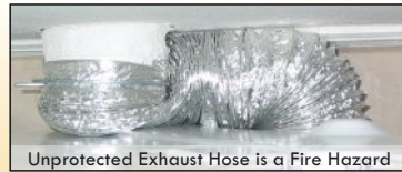
Unprotected Exhaust Hose is a Fire Hazard
