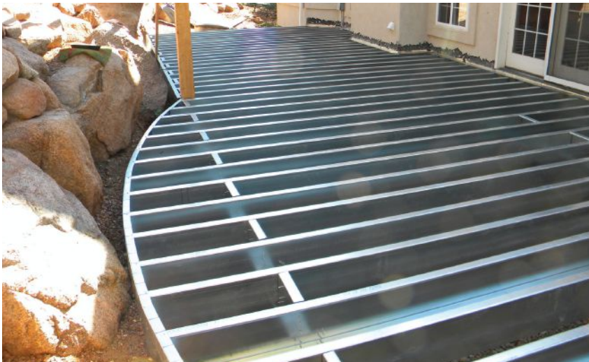
Figure 4. Complex framing can take longer with steel than with wood. For decks like the one pictured here, the steel has to be cut to length on site. Plus, complicated designs have a lot of screwed connections, which take longer than gun-nailed wood connections.
