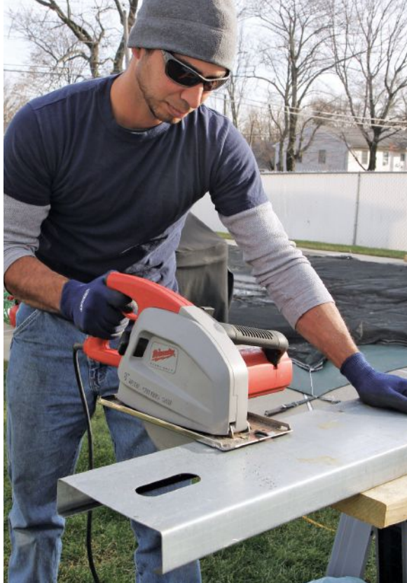
Figure 7. A specialized steel-cutting saw makes quick work of cuts and does a good job containing the hot chips of steel from the cuts.
