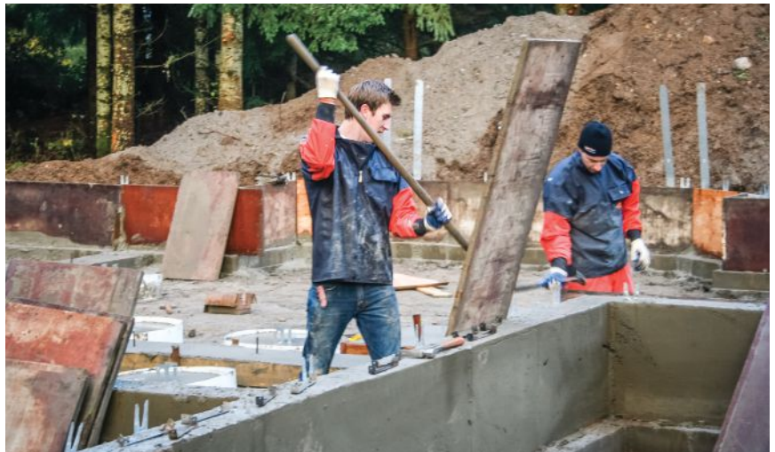
Figure 8. Workers scrape the panels clean as they strip the forms from the foundation. Later, they'll oil the panels before storing them.
