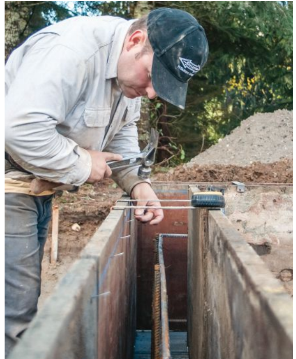
Figure 5. A reference line snapped within the top inch or two of the forms indicates the elevation of the top of the wall. The author tacks a 3D finish nail every 12 to 16 inches along the snapped lines to make them easier to find during the pour.
