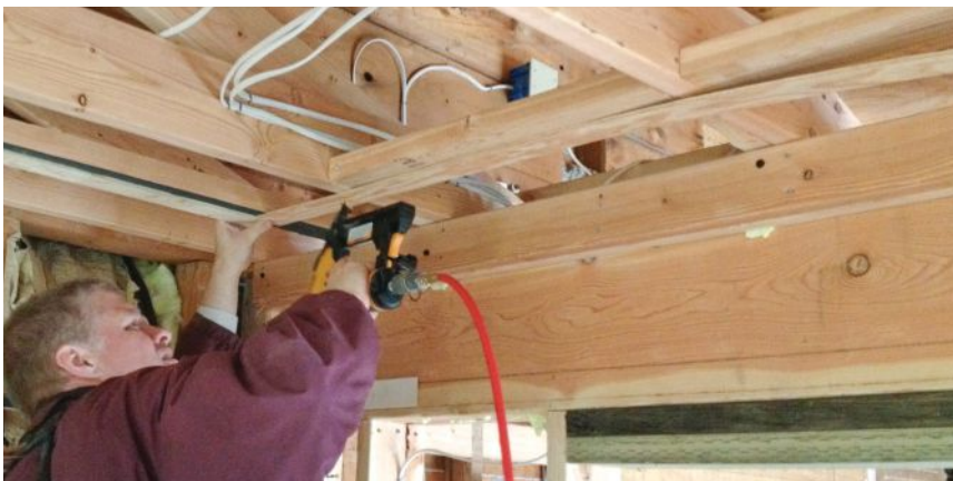
Figure 3. To bring the \frac{5}{8} -inch ceiling drywall, \frac{1}{2} -inch wall drywall, and \frac{1}{4} -inch flexible drywall that would be used to form the cove into the same plane, \frac{1}{4} -inch plywood furring strips needed to be attached to the blocking.
