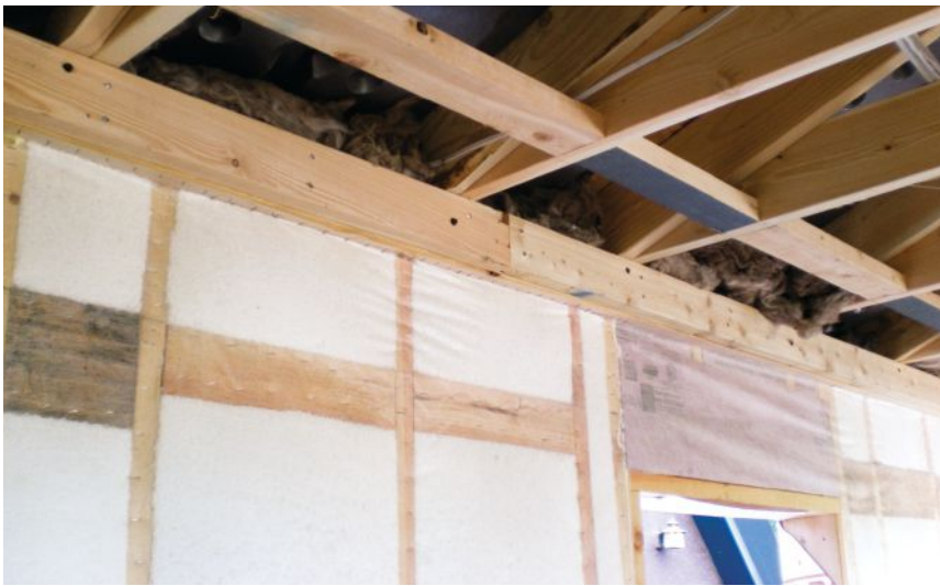
Figure 2. To provide a solid attachment point for the prefabricated arches, the author installed rows of blocking between the wall and ceiling framing. The blocking is centered 12 inches from the wall/ceiling intersection, and also provides good backing for drywall.
