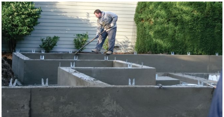
Figure 9. Before installing the mudsills, the author uses a scraper to smooth out any trowelling irregularities on the top of the stem walls.
