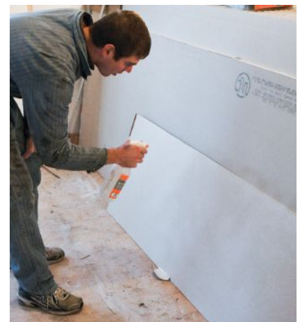
Figure 6. Workers sprayed both sides of each panel with a mister. Allowing the wet panels to sit for a few minutes before installation increased their flexibility even more, making it easier to form the flexible drywall to the 12-inch radius of the cove.
