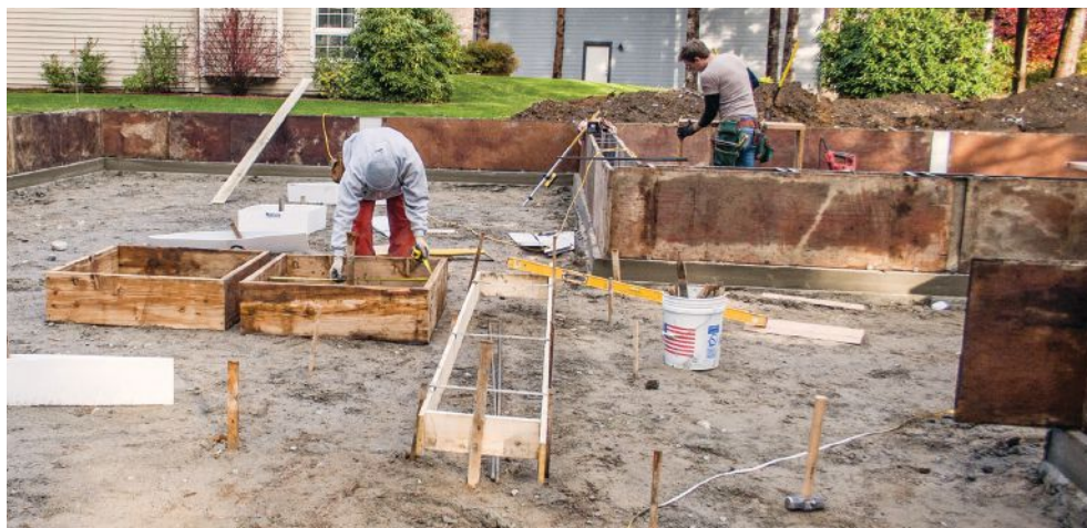
Figure 10. Here, the author's crew has formed footings for an interior shear wall and for several large piers that will support point loads from the roof.
