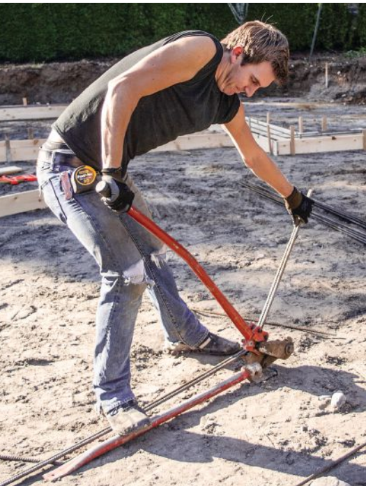
Figure 7. Most contractors cut and bend rebar on site, as shown. An option in some areas is to have a local metal shop pre-cut and pre-bend the rebar.
