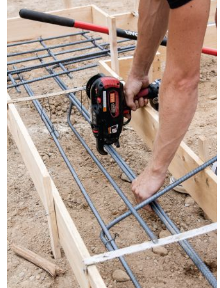
Figure 6. Companies that do production foundation work may want to consider the Max cordless rebar tier ( maxusacorp.com ), which automatically makes a tie in less than a second.
