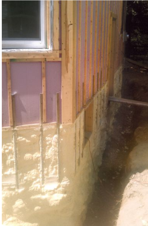
Most foundations in the DER houses needed waterproofing anyway, creating an opportunity to add foam to all of the foundation exteriors. Most received a double layer of rigid foam (far left); in two cases, spray foam — which served as a drainage plane — was the better choice (left).
