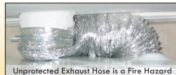
Unprotected Exhaust Hose is a Fire Hazard
