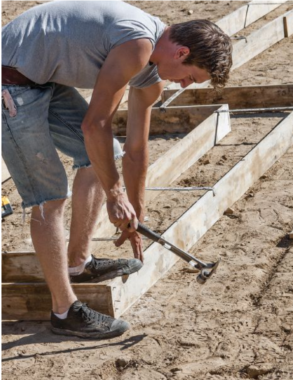
Figure 2. Footing forms are fastened together at the corners with duplex nails; 16-inch metal spreaders keep the sides properly spaced.
