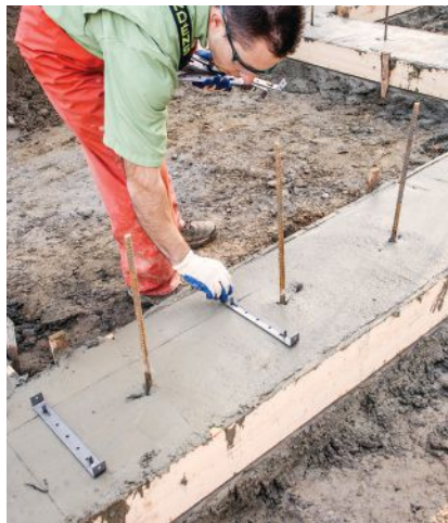
Figure 13. Form clips are set every 16 to 24 inches along the snapped layout lines. The author holds them in place with 1½-inch Teco nails pushed into the wet concrete; even if rain washes the lines away, the clips will still be in the right position for the stem-wall forms.
