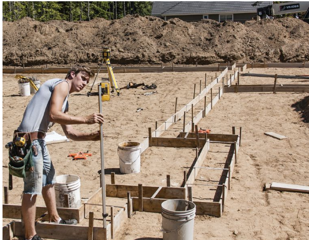
Figure 4. A single crew member can level the staked forms using a rotary laser. The receiver included with the Stabila LAR250 kit used by the author indicates distance from grade in \frac{1}{16} -inch increments.
