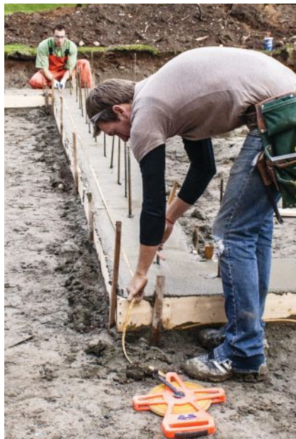
Figure 12. Workers lay out the stem walls on the footings, snapping lines while the concrete is still soft.
