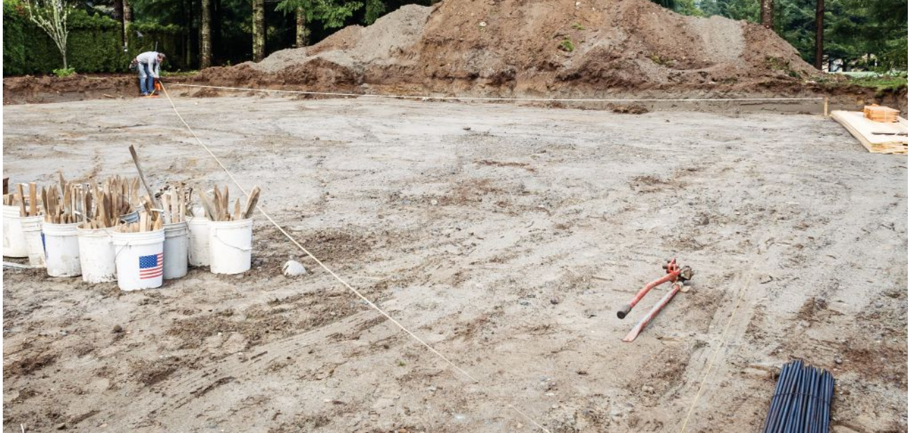
Figure 1. When laying out the footings, the author determines diagonal measurements using the rise/run function on his construction calculator, then refers to those measurements to verify that corners are square. The stretched string on the right-hand side of the photo indicates the outside edge of the first set of footings.
