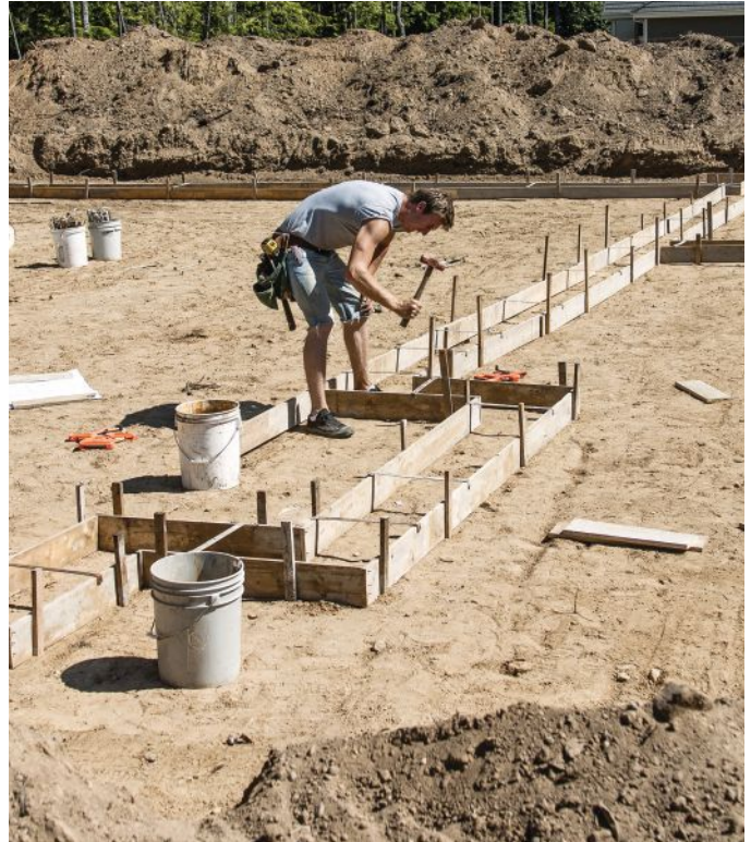
Figure 3. Either metal or wooden stakes can be used to hold the forms in place. In hard ground, a metal stake can be used to “predrill” holes for cheaper wooden stakes.
