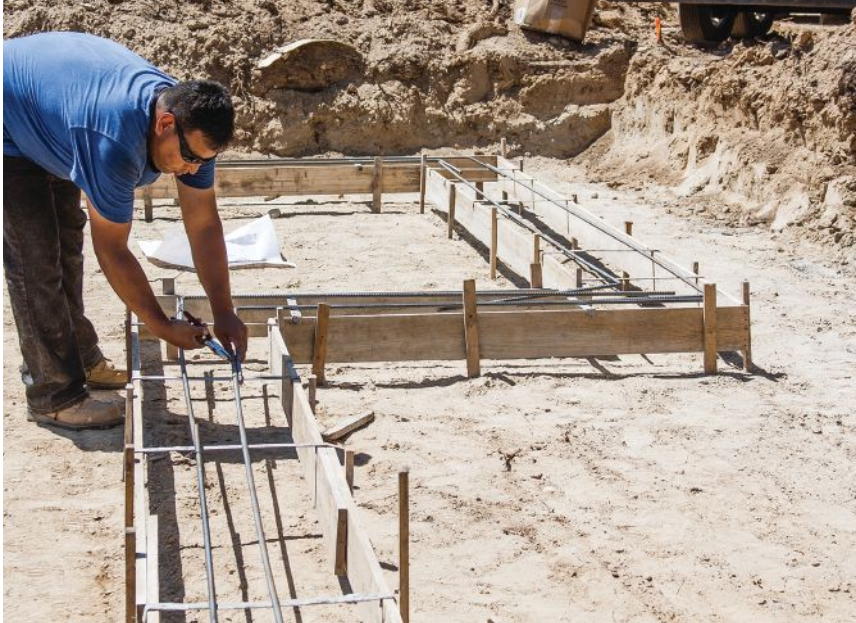
Figure 5. Tying the rebar together on top of the spreader cleats makes it easier to get the overlaps and spacing right. Afterward, the spreaders can be temporarily removed and the rebar dropped in place.
