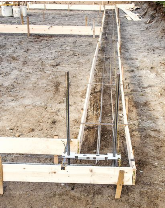
Figure 8. To place the rebar at the proper depth in the footing, the author suspends it from the spreader cleats. Here, he's also used a template to accurately locate the 1-inch-diameter all-thread rod needed for an iLevel shear-wall brace.
