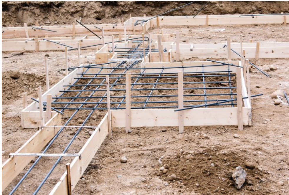
Figure 9. Areas in the footings that must support point loads are reinforced with rebar following the engineer's specifications.
