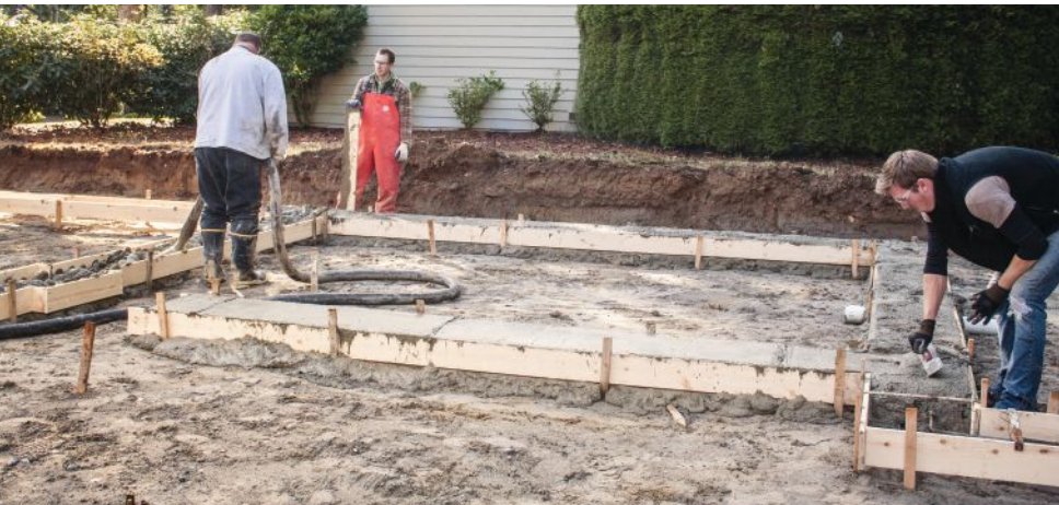
Figure 11. As the line pump operator fills the footing form, a crew member follows behind and screeds the concrete level. A second worker then trowels the footing smooth.
