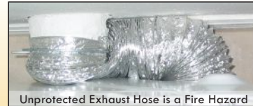
Unprotected Exhaust Hose is a Fire Hazard
