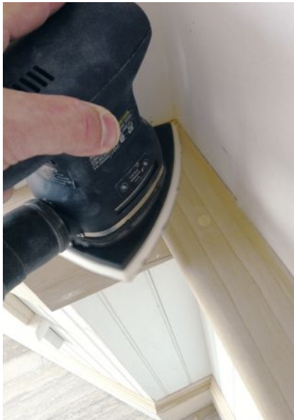
Figure 1. The author sands new trim-work with 120-grit paper before filling holes and priming. Good dust collection streamlines the process.
