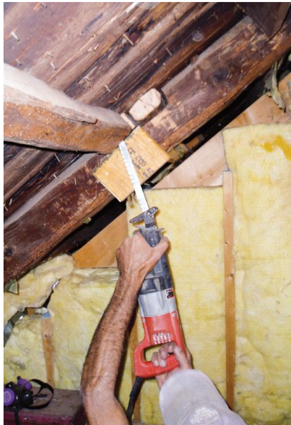
Figure 2. The original undersized purlins were small-dimensioned pieces of timber hewn flat on two sides, with some of the bark left on. Their ends were carefully cut free of the rafters, creating space to insert LVL sisters.
