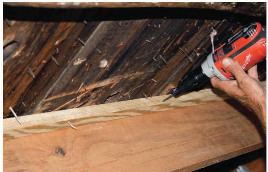
Figure 4. A 1½-inch by 1½-inch nailer fastened alternately to the purlins and the roof boards stiffens the assembly against racking without penetrating the existing roof shingles.
