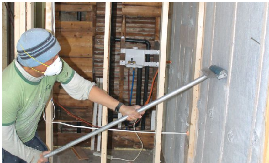
Figure 5. Filled cavities are compacted with an aluminum roller to avoid bulging drywall. A quick pass of the hand is enough to confirm that the insulation lies flush with the framing.
