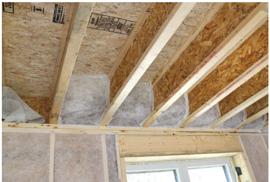
Figure 7. A strip of netting between a top-plate nailer and the facing joist makes it possible to dense-pack this area of the band joist (top). Netting stapled between the joist ends is filled with cellulose to form insulating and air-sealing "pillows" (above).
