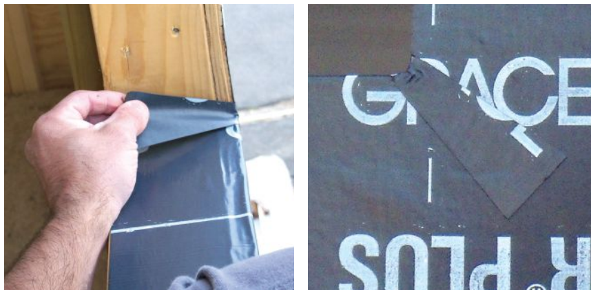
Figure 4. One end of a bow tie is adhered to the flashing membrane outside the opening, the other half folded to the inside (left). When applied correctly, the narrow center section will turn neatly up the corner of the opening (right).
