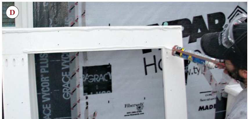
Figure 10. The backs of the prepared sill and casings are drilled for pocket screws (A). Facing surfaces are then coated with PVC cement and temporarily clamped together while the screws are driven (B). Next, the completed trim assembly is drilled for the deck screws that will fasten it to the framing, and caulked on the back before being lifted into place (C, D).
