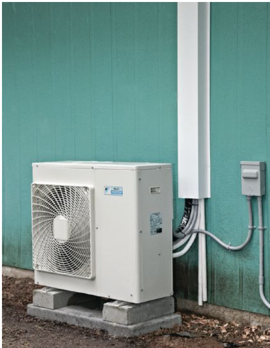
Figure 8. Refrigerant lines and wiring on the exterior wall are protected with a vinyl or sheet-metal cover. Condensate drain tubes are visible at lower right.
