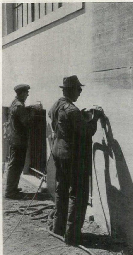
Fig. 1. Giving a surface finish to a concrete factory with grinding wheels made for the purpose
