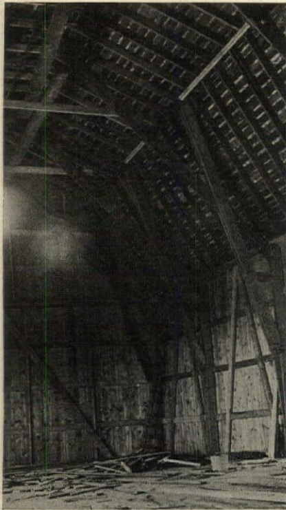
Fig. 4. Another modification of Shawver truss showing purlin post No. 5 brought into wall half way between main plate and floor
