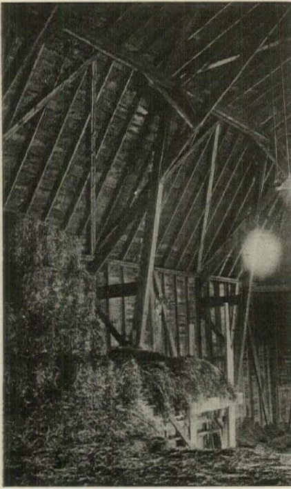
Fig. 2. One of the first Shawver truss barns to be built in the East
