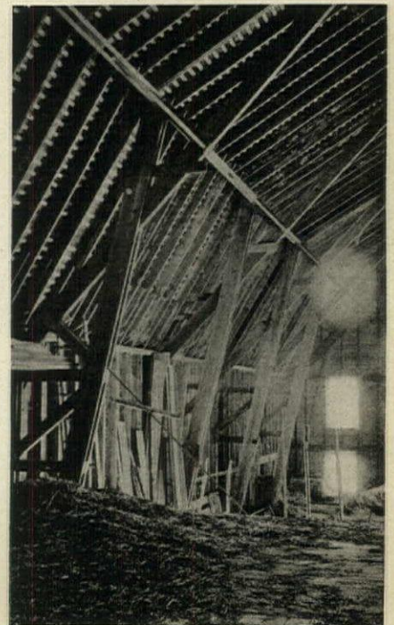
Fig. 3. Shawver truss with Nos. 2 and 3 omitted. Auxiliary hay floor suspended by iron rod so truss is doing double duty
