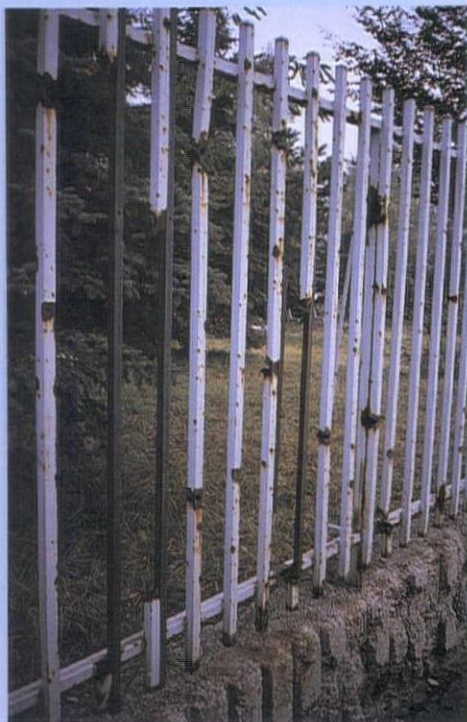
Fence around barracks, re-arranged by explosions.
