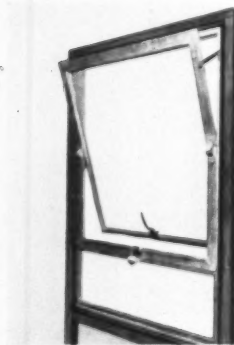
1. Open for ventilation
