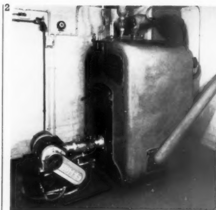
A typical domestic installation.
