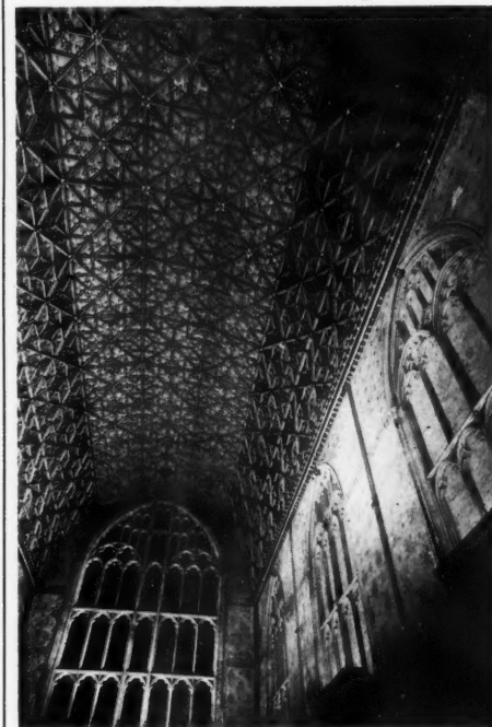
9, the roof of Canterbury Chapter House, with concealed lighting by Drake & Gorham—see Booklets Received, page 426.
