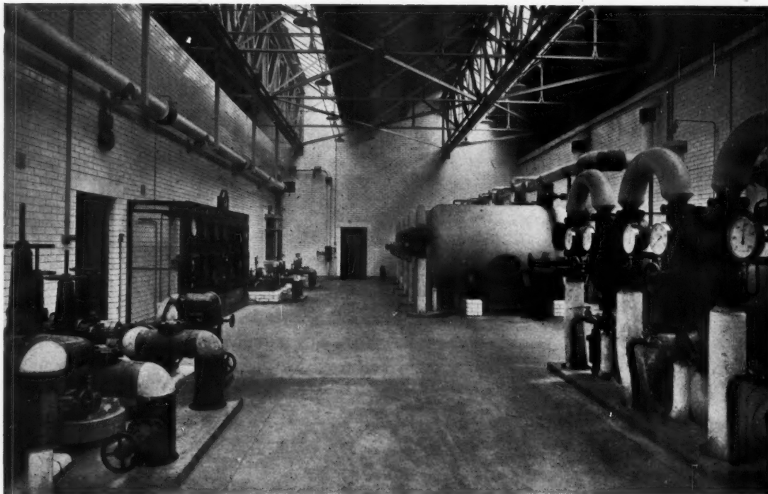
Calorifier and Pump Chamber by Hadens. 60 million B.Th.U. per hour.
