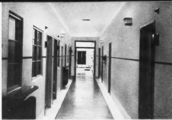
INDIRECT LIGHTING FROM WALL BRACKETS. Architects : Bromley, Cartwright & Waumsley, A.L.R.I.B.A.
