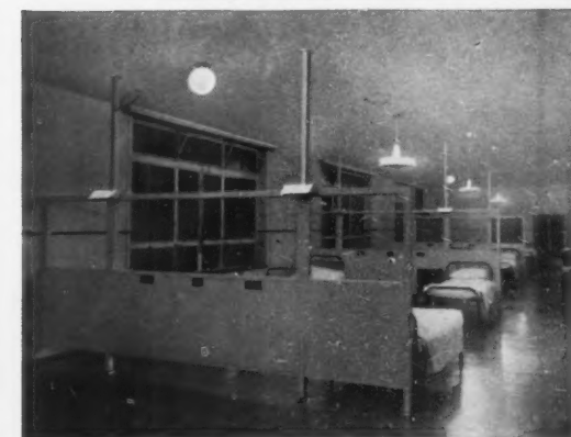
PENDANT AND BED LIGHTING IN A HOSPITAL. Architects : Bromley, Cartwright & Waumsley, A/L.R.I.B.A.
