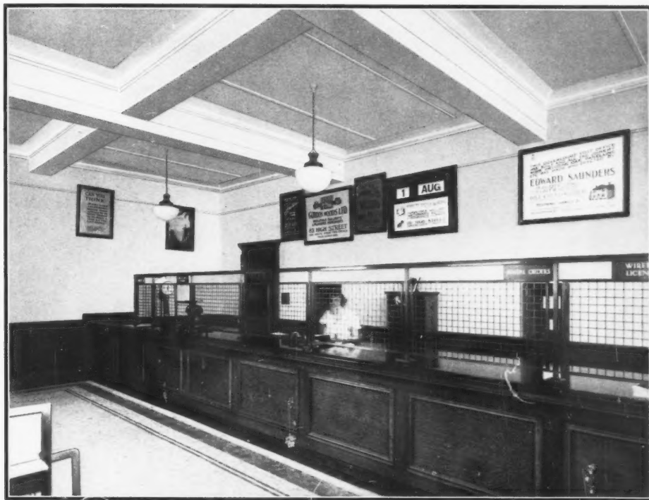
Illustration shows No. 35 Ideal Rayrad fixed on ceiling in a Post Office The steel surface plates have been drilled to accommodate the electric light fittings
