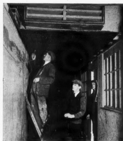
Air conditioning, like every other boon, brings trials and troubles in its train. Moving air sets up vibrations in the metal trunking with a resultant "drumming" sound. The illustration shows how the problem was dealt with in the corridors of Broadcasting House, London. As is clearly indicated, the ducts are lined with an absorbent material producing very successful results. Whilst the ordinary office building would neither require such a volume of air change to be carried along its corridors, nor the need for such a degree of sound elimination, it is desirable in the interests of quietness, that all ventilation ducts in the public or letting part of office blocks, should be insulated.
