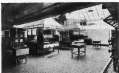
The kitchen of Messrs. Harrods' Georgian restaurant is equipped with gas and steam apparatus in enamel and stainless metal.
