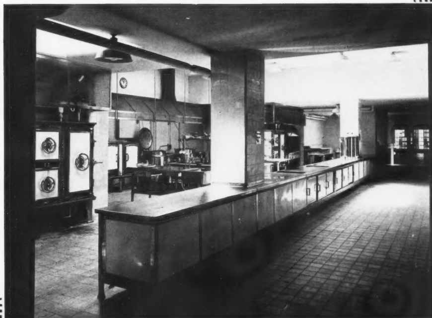
Part of the main kitchen of the Royal Masonic Hospital, Ravenscourt Park. Architects: Messrs. Sir John Burnet, Tait & Lorne. Consulting Engineer: Stinton Jones, Esq. The whole equipment is of special hygienic finish, viz: the use of stainless steel, mottled enamelled surfaces and chromium plating. (Photograph by courtesy of The Architectural Review .)
