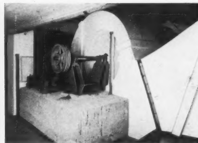
100 One of the fans and fan motors of the Broadcasting House concert hall air-conditioning equipment. (Note vibrating insulating joint.)
