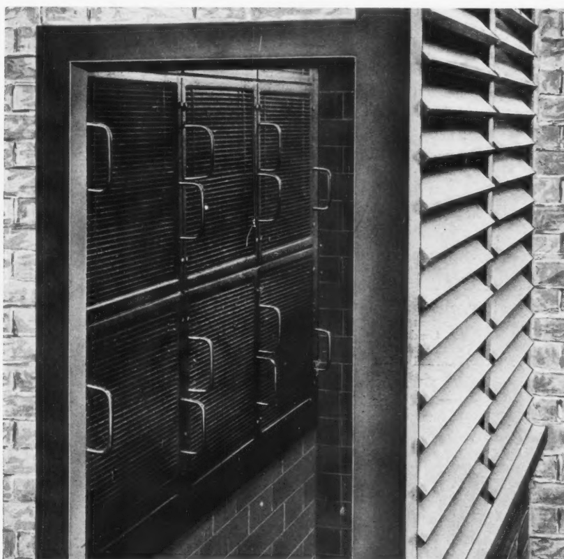
An AIR FILTER on the roof of a large London store, formed by a number of units bolted together. The louvred frame is a protection from the weather. Designers and Engineers: Ozonair.
