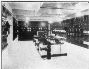
CONTROL ROOM, REGENT POLYTECHNIC, LONDON
