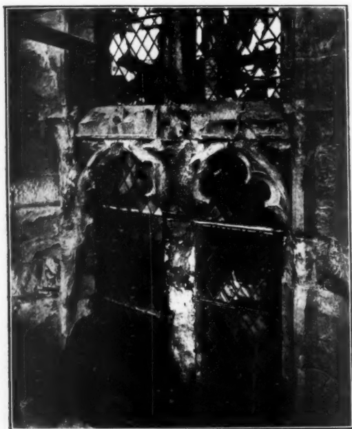
DECAYED LANTERN WINDOW.
