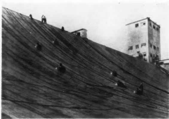
"HUMAN-FLY" WELDING OPERATORS AVERAGE 40 TO 50 FEET OF LAP WELDS PER HOUR ON 12 GAUGE STEEL IN FABRICATING SUSPENDED STEEL ROOFS ON GRAIN ELEVATORS AT ALBANY, N. Y. EACH OPERATOR EMPLOYED A SHEAVE BLOCK AND FALL TO HOIST HIMSELF.
