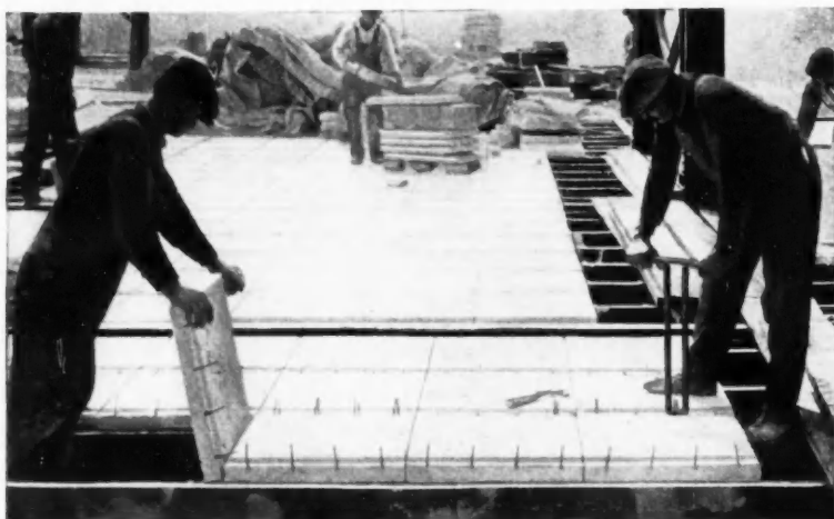
Laying Floor Slabs on top of steel members and tying steel rods together.
