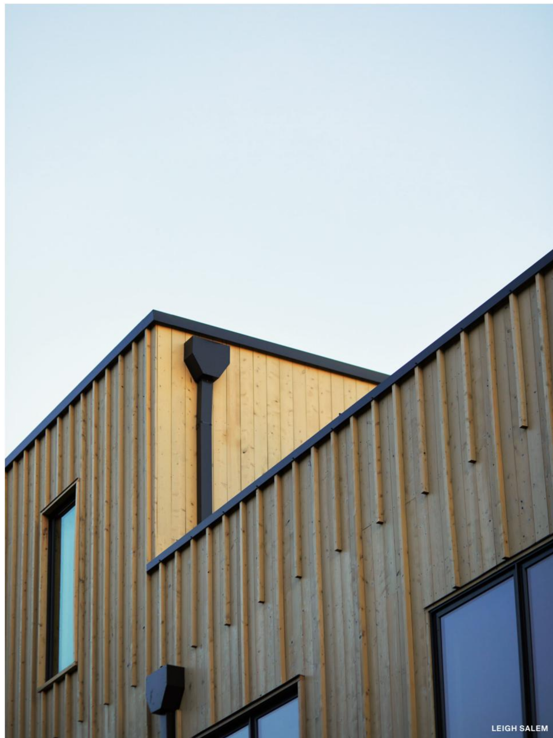
The number of units in 440 West Kelly, designed by Post Company, was scaled back because of objections over density in Jackson.
