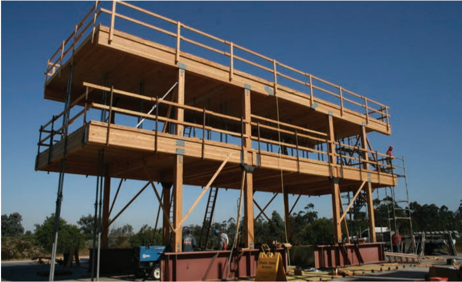
A two-story prototype is tested on the world's largest shake table at the University of California San Diego.
