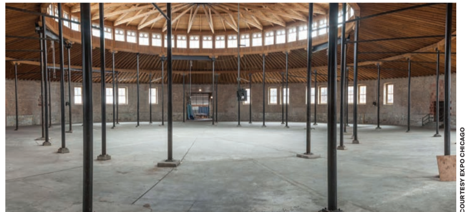
Unable to convert the Roundhouse into whitewall gallery space, DuSable opted to leave the interior in its original timber and iron form.
