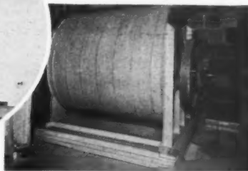
Above—FANS FOR AIR-CONDITIONING in the Codman Square Theatre, Dorchester, Mass. Armstrong's Vibracork is employed to absorb vibration—caused by the fan and quiet unwanted noise.
