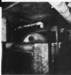
Above—BOILER ROOM in the Tyler Hotel, Louisville, Kentucky. Fuel costs are cut by insulating boiler and drum settings with Nonpareil Insulating Brick.
