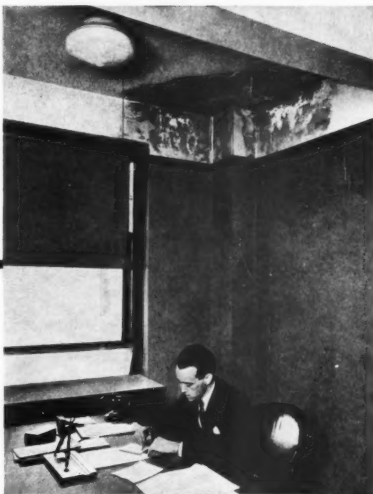
Interior Damage caused by wall seepage. It's cheaper to prevent this in the beginning.
