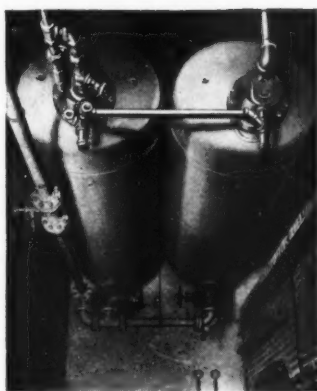
Two of the Everdur Tanks in the Canada Life Assurance Building, Toronto. Architects, Messrs. Spoatt & Rolph, Toronto. Each tank measures 36 in. by 96 in., holds 424 gals. and is made of 0.187 gauge Everdur, acetylene welded.
