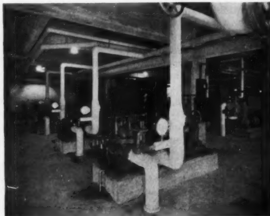
HOUSE PUMPS AND SURGE TANK IN BASEMENT "C"
