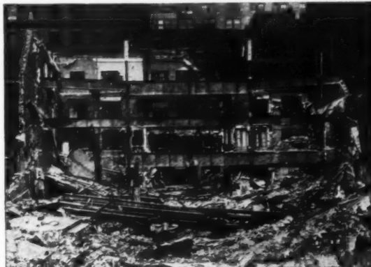
FORREST THEATRE, PHILADELPHIA, ERECTED IN 1905. DEMOLISHED IN 1927. STEELWORK WAS FOUND TO BE FREE FROM CORROSION
