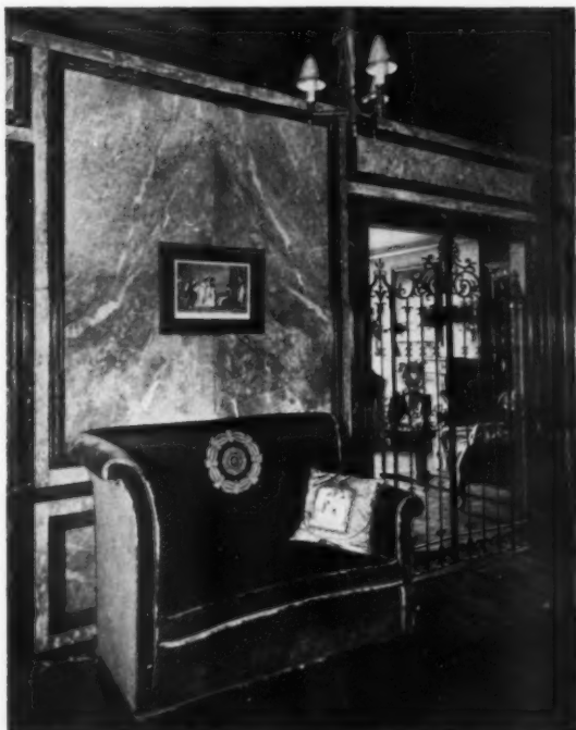
WHILE DECORATIVE, MARBLEIZED WALLS LACK THE STRUCTURAL SIGNIFICANCE THEY SHOULD SUGGEST UNLESS APPROPRIATELY DESIGNED AND DETAILED
