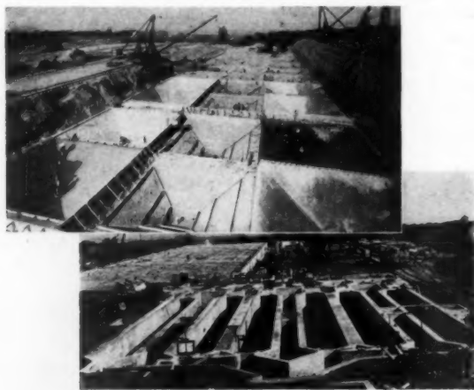
Rochester Sewage Disposal Plant, Rochester, N. Y.
