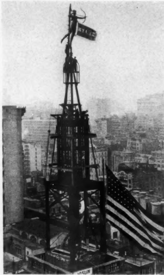
TOWER FRAMEWORK STRIPPED OF ITS COVERING AND BRACED. THE STEELWORK WITHIN THE BRACED AREA WAS CORRODED AND IN MANY PLACES THE CIRCULAR STEEL DRUMS WERE PRACTICALLY DESTROYED. NOTE THE GIN-POLE SET FOR LOWERING THE STATUE OF DIANA TO THE MAIN ROOF FROM WHENCE IT WAS LATER LOWERED TO THE STREET AND PLACED IN STORAGE
