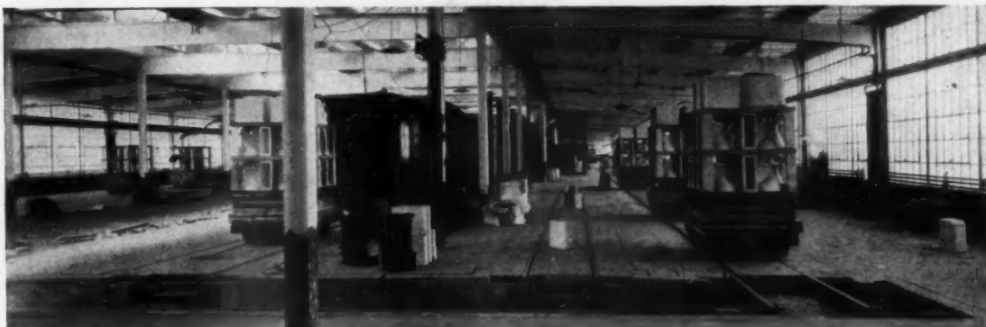
EXIT END OF THE GLOST KILN, SHOWING POTTERY ON THE TRUCKS, TRANSFER TRACK AND RECORDING INSTRUMENT ROOM NEAR THE CENTER OF THE KILN
