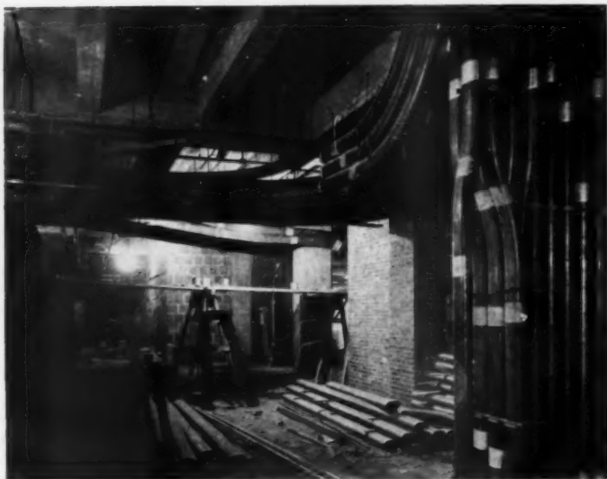
A PORTION OF THE PNEUMATIC TUBE SYSTEM
