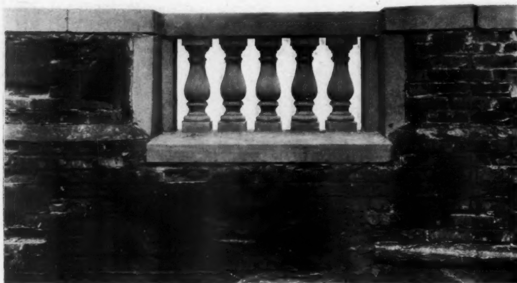
View looking north. In the lower part of the second, third and fifth balusters (counting from the left) cracks are clearly shown which extend entirely through them. The bases and tops of the balusters are tightly doweled to the coping and sill stones. These cracks indicate the uplifting force exerted by the frost in raising the coping stone
