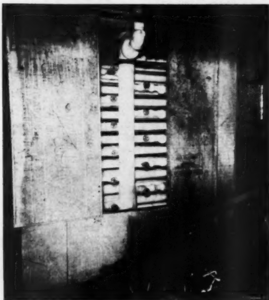
VIEW OF THE COIL BUNKER THROUGH WHICH THE AIR IS PASSED OVER BRINE COILS AND COOLED AND DRIED BEFORE ENTERING THE COLD STORAGE ROOMS
