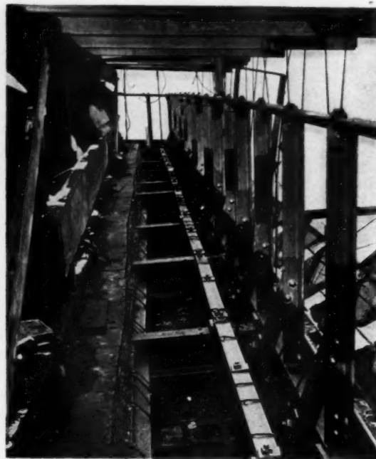
The original structural steel was corroded to band iron thickness and had to be replaced. Some of the original beams that were properly protected from the water which entered through the vertical joints were not corroded
