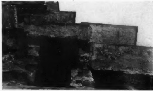
THIS IS NOT A PICTURE OF THE ENTRANCES TO SOME ANCIENT CAVERNS. IT IS A PORTION OF A CORNICE AND PARAPET WALL OF A MODERN AMERICAN BUILDING. THE MASONRY WORK WAS DONE IN A MOST CARELESS AND SLIPSHOD MANNER. THIS COULD NOT HAVE HAPPENED IF COMPETENT SUPERVISION AND INSPECTION HAD BEEN EXERCISED WHILE THE BUILDING WAS UNDER CONSTRUCTION
