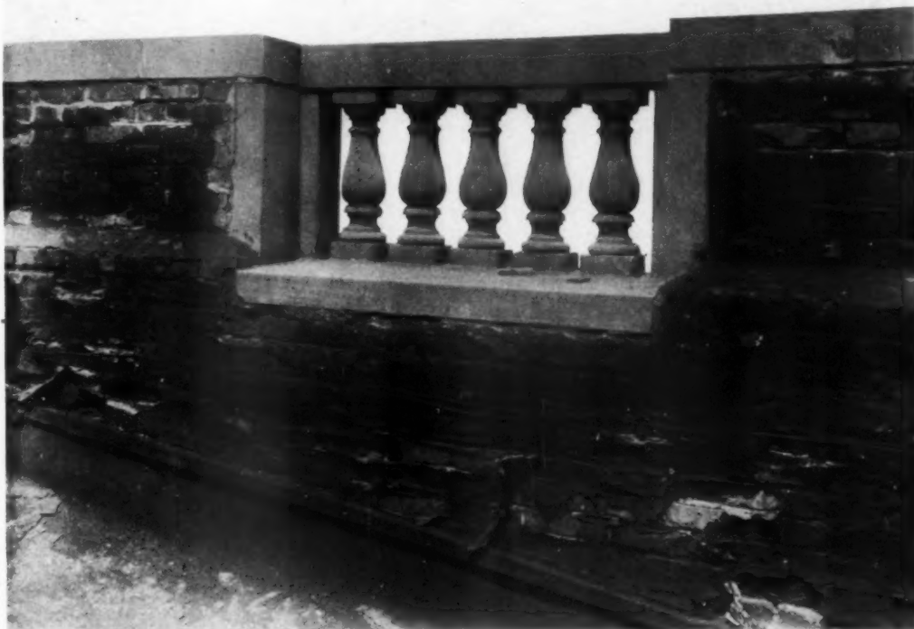
View looking north. The spalled brick and destroyed waterproofing as well as the open joints in the stonework are clearly shown. The face of the right hand jamb stone of the balustrade projects beyond the face of the coping stone above it and doubtless this projection provided a shelf for the accumulation of water and frost which eventually displaced the stones
