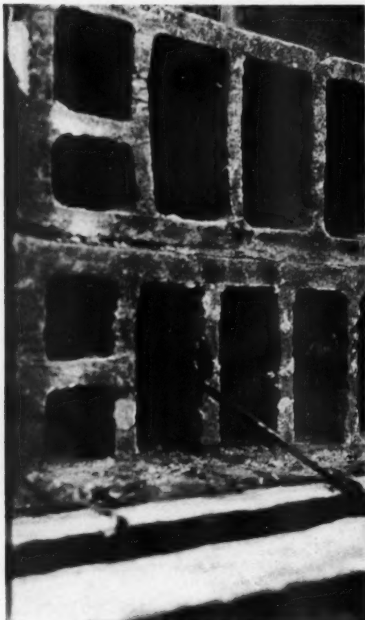
The structural steel supports and the anchors are both badly corroded. The terra cotta is not backed up or filled and the improperly made vertical joints permitted the free access of water
