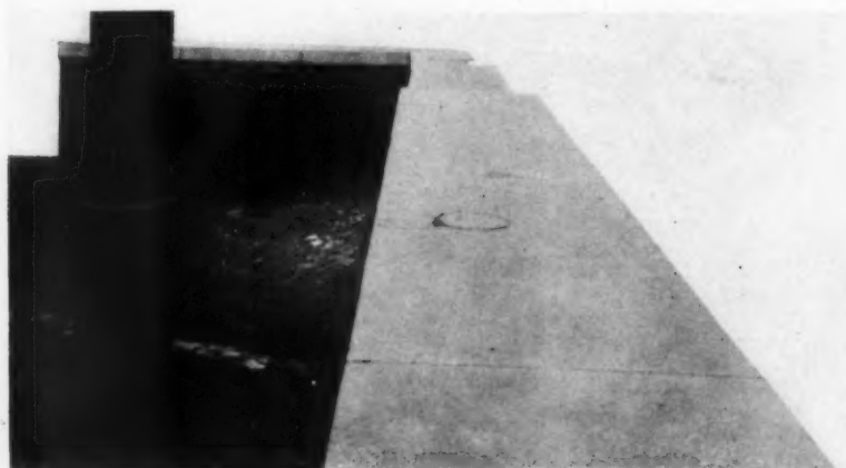
VIEW LOOKING WEST. THE UNEVEN LINE OF THE COPING STONES NEAR THE RETURN WALL IS OVER ONE OF THE STONE BALUSTRADES
