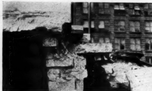
On opening up the cornice, the coping was found to be improperly set with no apparent care given to securing tight vertical joints
