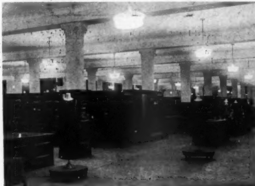
Effective installation of white glass semi-indirect luminaires in a department store. One outlet is provided in the center of each bay, the spacing being 16'-0" x 30'-0"
