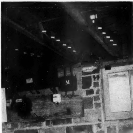
KNOB AND TUBE. ARRANGEMENT OF SWITCHBOARD AND METERS IN BASEMENT. THE OPEN WIRES IN CEILING EXTEND TO ALL PARTS OF THE BASEMENT, OFFERING OPPORTUNITY FOR TAMPERING BY AMATEURS
