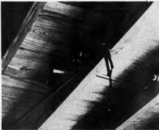
KNOB AND TUBE. WIRING TO COMBINATION FIXTURE IN KITCHEN CEILING
