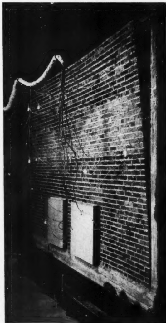
Fig. 13. Unexposed side of 13" solid unrestrained Eastern surface clay brick wall after 6-hour fire test, Test No. 10
