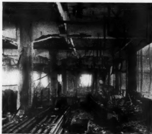
Fig. 3. An interior view of an apparatus room after the fire
