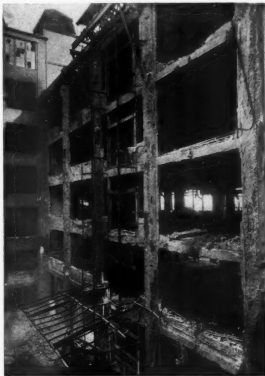
Fig. 1. Appearance of walls on Interior Court after the fire in the Sarotti Chocolate Factory, Berlin, Germany
