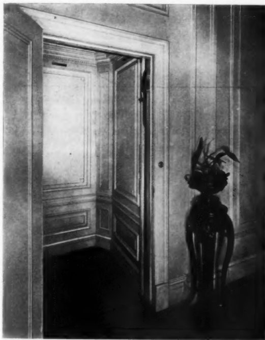
ANOTHER INSTALLATION SHOWING THE SAFETY DOOR LOCK. BANK OF OPERATING BUTTONS CAN ALSO BE SEEN ON THE RIGHT SIDE OF CAR
