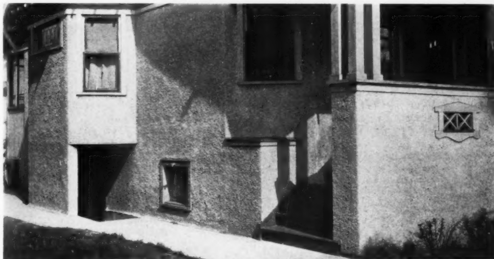
A residence in Oak Park Ill., photographed 62 months after completion. A marble-finished magnesia cement stucco applied to sheathing board having dovetailed grooves on its face. Note the color and texture
