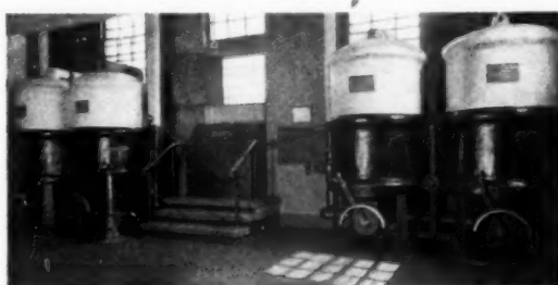
View of the filters, two of which are used for filtering the polluted water drawn from the pool. The other two filters are used in case of emergency and to filter the fresh water as it is used.
